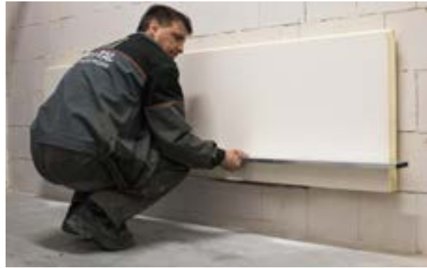
Stage II. c) Installing and laying subsequent boards in the first row.
