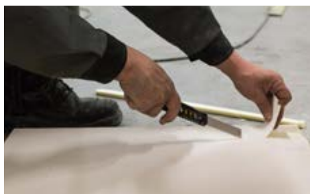
b) Removing the facing from the board section joined with the face of the lateral one.
