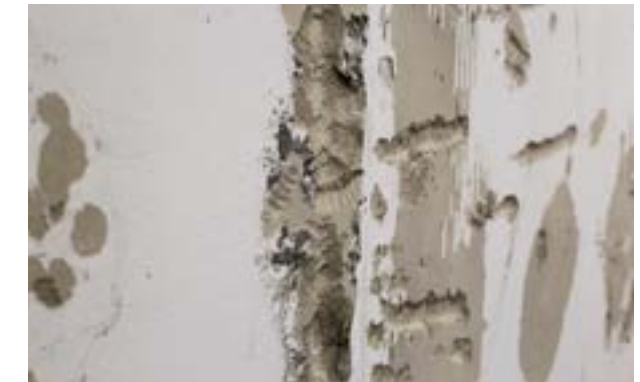
Photo 02. Matter remaining after previous finish layers were removed.
