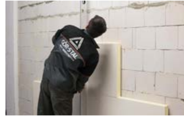
Stage III. a) Installing and positioning the second and third board rows.
